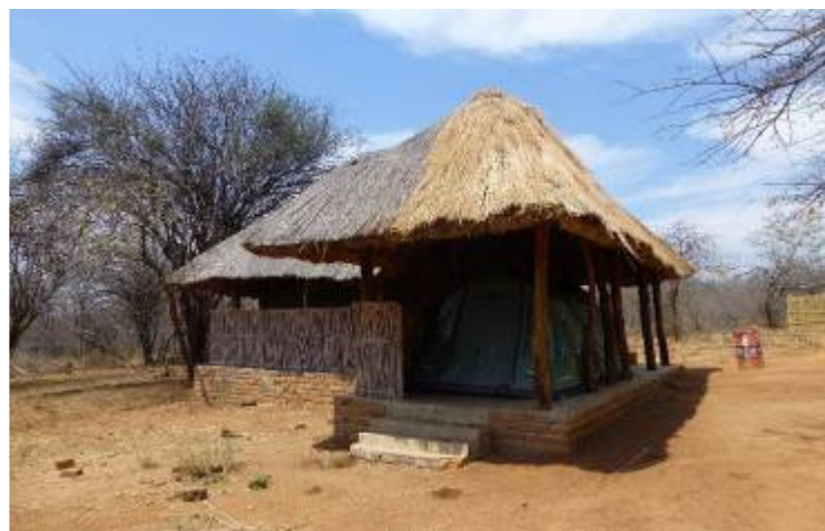
A part of this roof was destroyed because termites found their way into it
